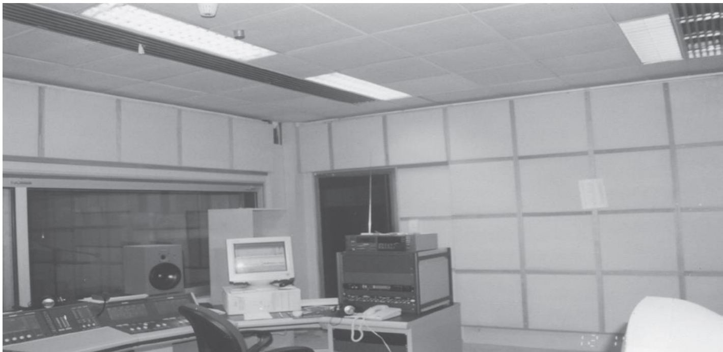
Sharjah T.V. Station - F.M. Radio Studio, BETEC CAD. Acoustic Panels for Studio Applications - Model: AP - AB-42-50 Size 600 x 600 mm
