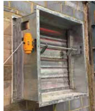
Damper Condition after 4 Hrs
