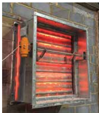
Damper Condition after 2 Hrs
