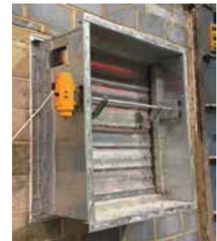
Damper Condition after 4 Hrs
