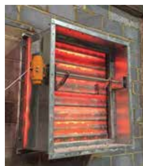
Damper Condition after 2 Hrs
