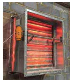
Damper Condition after 2 Hrs
