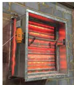
Damper Condition after 2 Hrs
